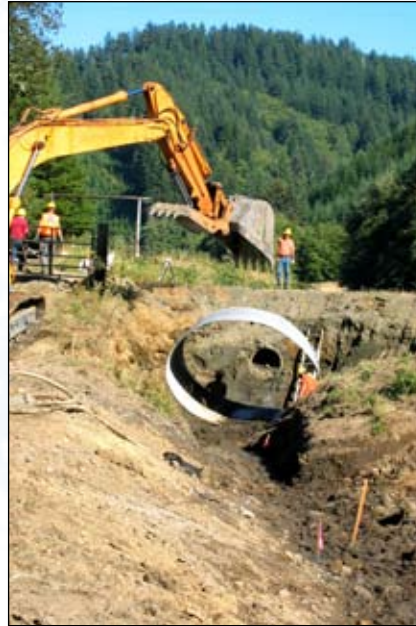
The Siuslaw Stewardship Group uses stewardship contracting to restore natural watershed processes, such as repairing or replacing culverts for safe fish passage.
